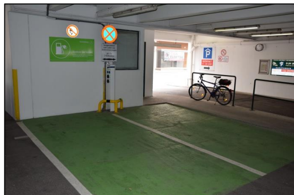
Figure 2: Charging station with ram protection installed in the middle between two parking spaces and corresponding signage of the charging station and the associated parking spaces (Source: im-plan-tat)
