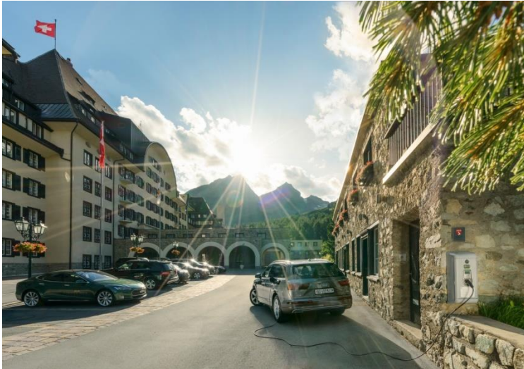
Figure 8: E-Grand Tour charging station (wall box), Source: https://www.presseportal.ch/de/pm/100059618/100803840
